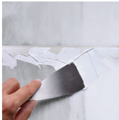
Once transition cap/corner guard is dry and secure, smooth and feather edges with dry-wall compound
